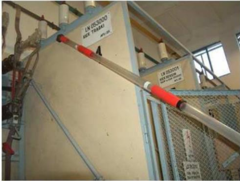
Fig. 16: Main suction tube H091-01 with extensions H091-02 and H091-04
