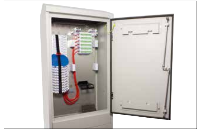
Point of Connection
