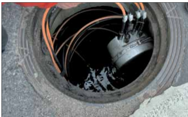
T240 closure in waterfilled man-hole
